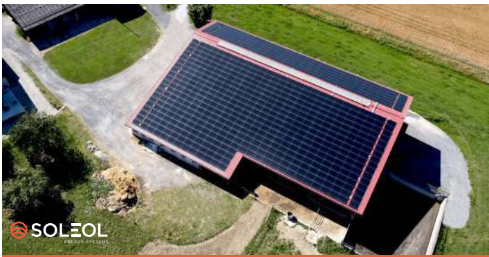
Project in Mézières Panels 646 – Area 1,212 m 2 – Power 252 kW
