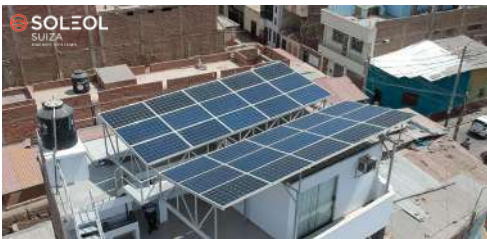
Project in Chiclayo Panels 30 - Area 49 m 2 - Power 8 kW
