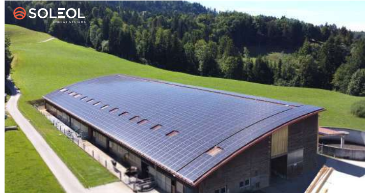
Project in Le Pâquier – Montbarry Panels 1'202 – Area 2,190 m 2 – Power 445 kW
